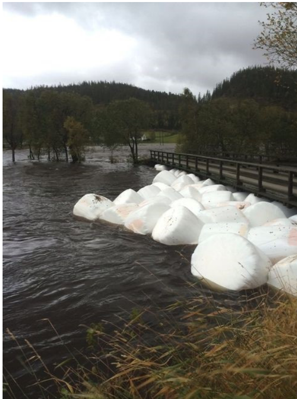
Figure 1: Obstructed spillway due to silo bales in Trondelag, Norway (Foto: L. Lia, NTNU).
