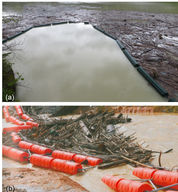
Figure 35: a) Broken Large wood barrier at the Montsalvens dam (Canton of Fribourg, Switzerland) during the 2015 flood event (Annex 2, Photo: Groupe E); b) Hydroelectric power plant Tulu Ter, Malaysia: Floating barrier with large volumes of large wood at the bypass tunnel inlet (Photo: Worthington).
