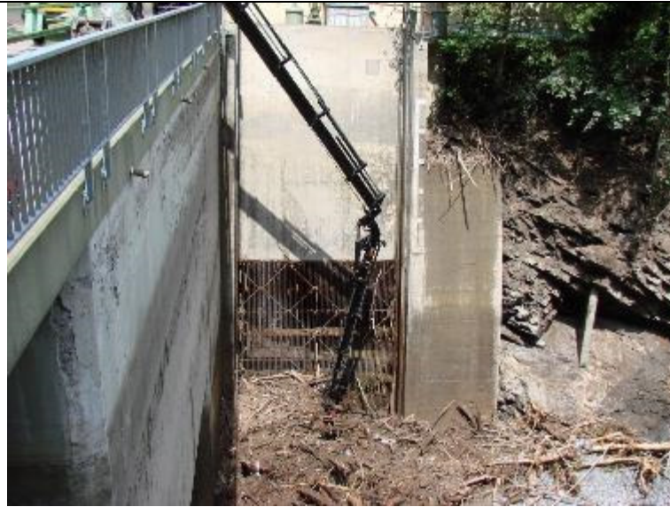
Figure 6: Mechanical removal of large wood at the water intake after the 2010 flood event (Source: ebs Energie AG)
