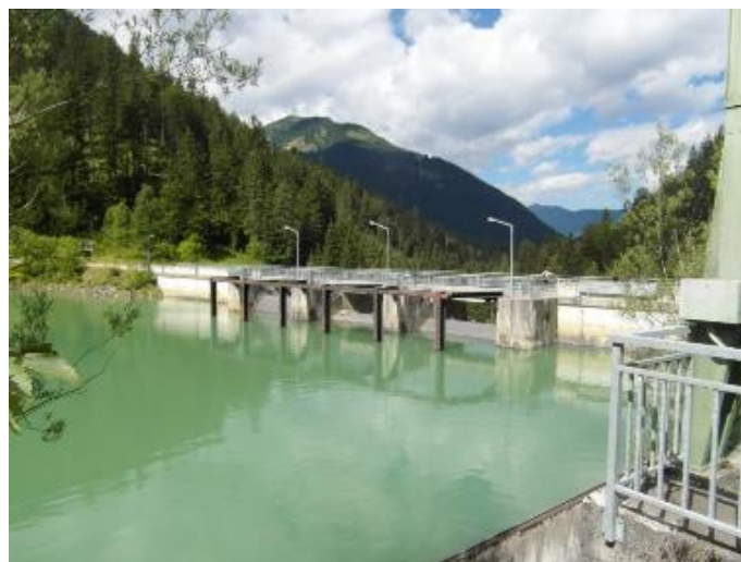
Figure 30: Upstream large wood rack at Rotlech Dam in Austria (Photo: Federal Ministry of Agriculture, Forestry, Environment and Water Management Austria).
