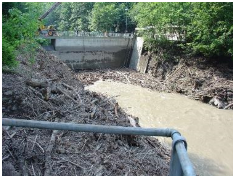
Figure 5: Outlet obstruction due to large wood after the flood in 2010 (Source: ebs Energie AG)
