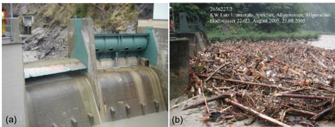
Figure 41: Gstins reservoir: (a) Dam spillway with two flap gates (Photo: VAW) and (b) obstruction during the 2005 flood event (Photos: Vorarlberger Illwerke AG).
