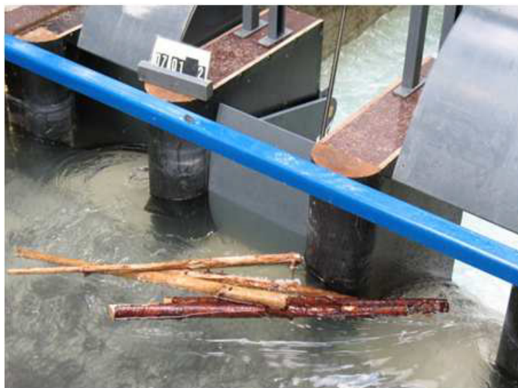
Figure 36: Obstruction at opened weir bays of a three-bay weir system (Hartlieb 2015)
