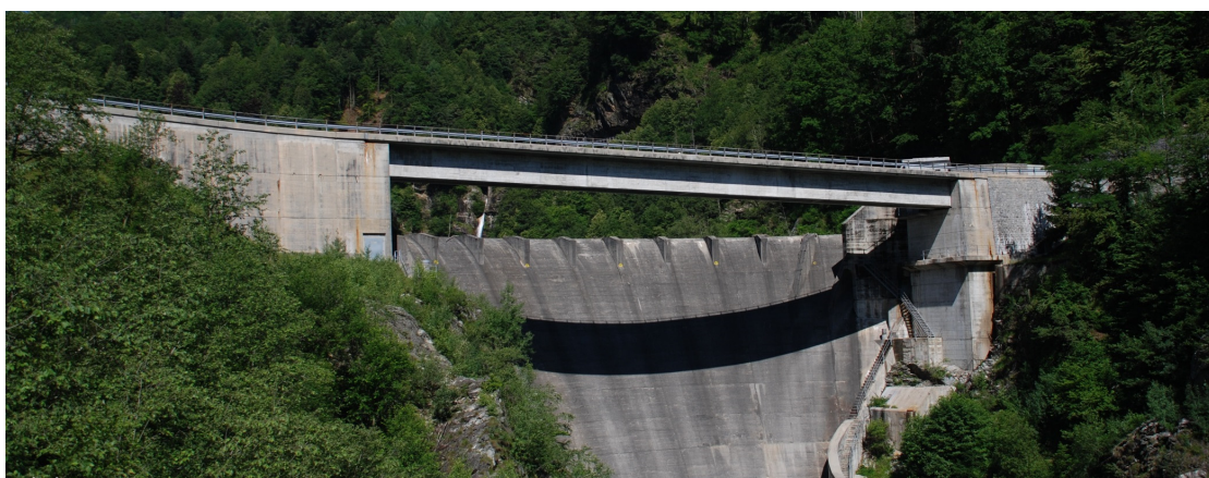
Figure 10: (a) Blocking of the dam spillway inlet structure (spillway with weir bridge) at the Palagnedra dam, Canton Ticino, 1978; (b) new dam spillway inlet structure without weir bridge (Photos: Ofima).
