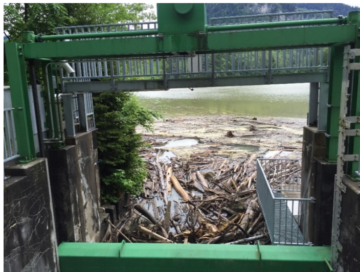
Figure 6: Current situation in a flood event; the obstructions risk remains unacceptably high
