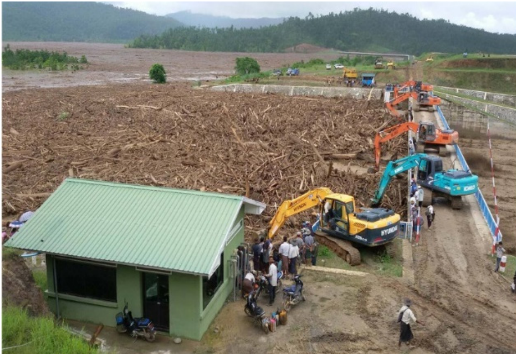
Figure 11: Removal of floating debris with excavators at the Yarzagyo dam, during the 2015 flood in Myanmar (Photo: M. Wieland).
