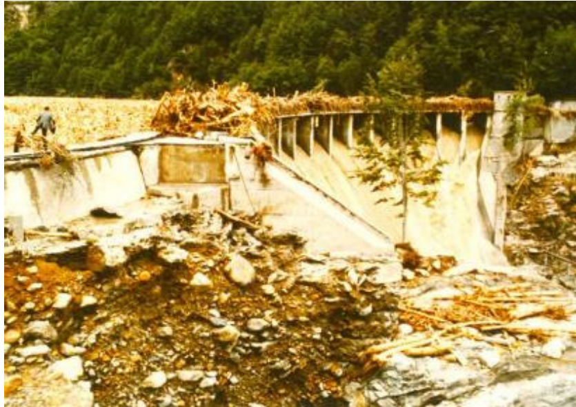
Figure 3: Dam spillway obstruction due to large wood and partially eroded core wall after the 1978 flood event (Source: Ofima)
