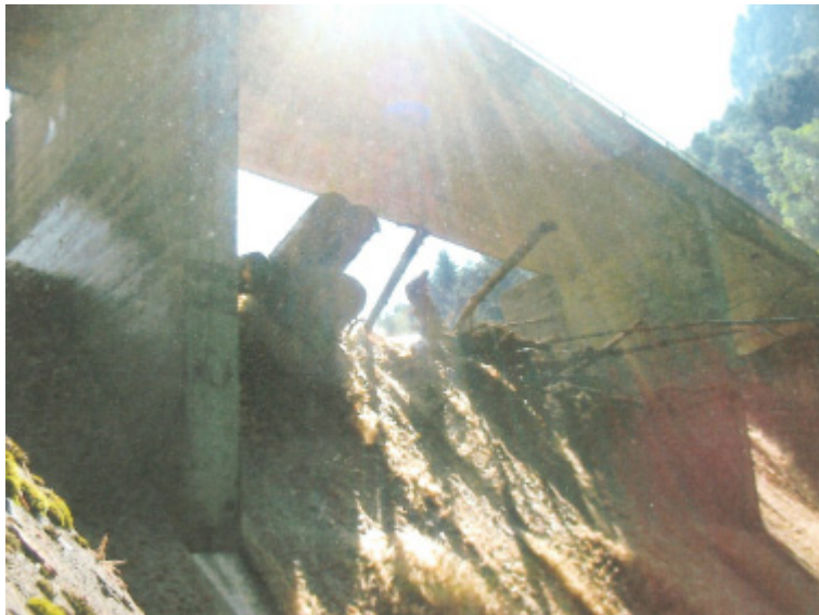
Figure 3: Dam spillway obstruction due to large wood during the 2005 flood event (Source: EW Nidwalden)
